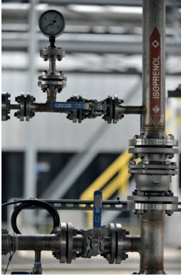
© Ban Seng – Transfer pipe for chemical products
