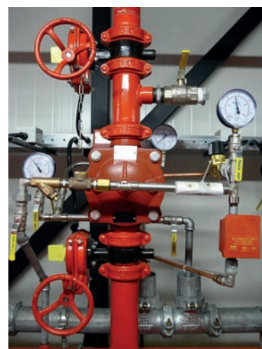
Fire system valves.
